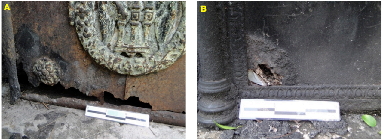
Figure 02 - Plane sheets from different mausoleums, which exhibit general corrosion, lacunae (A) and burned surfaces (B), due to mortuary rituals.
