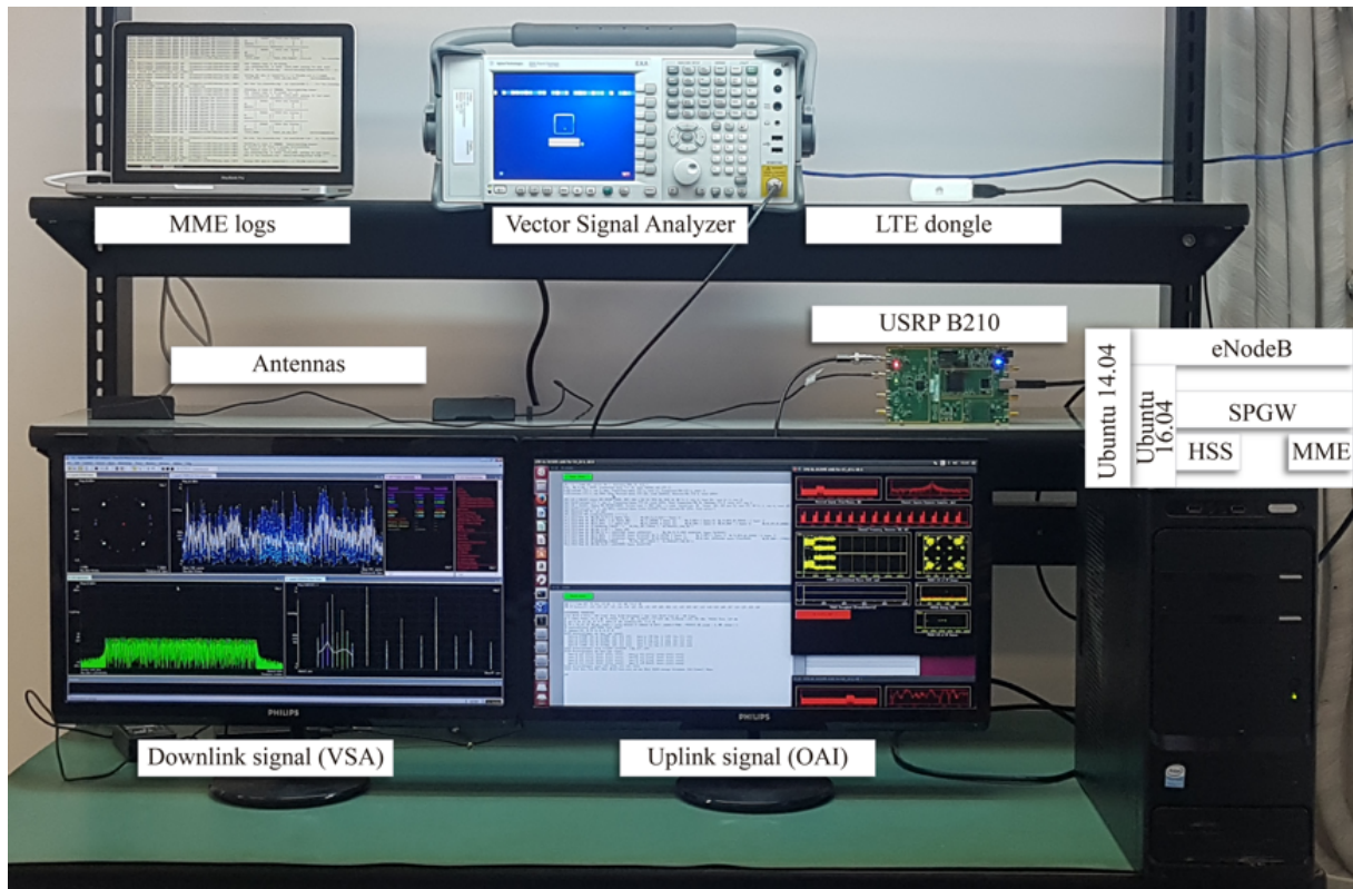
Figure 26 – Picture of the testbed used to generate the prototyped EPS network (4G) and experimenting with ICN.
