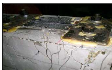
d) Ruptura do FRP (BM9)
