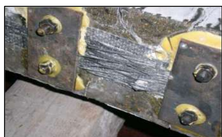
c) Ruptura do FRP (BM7)
