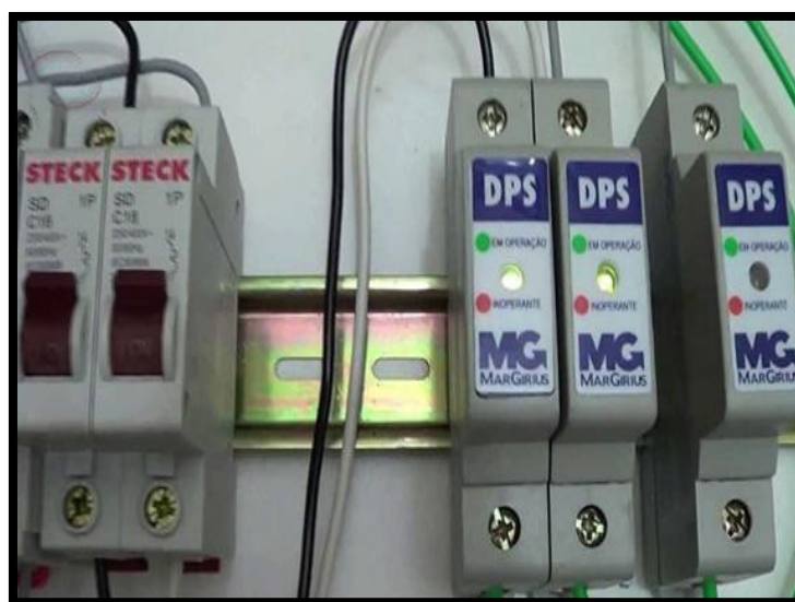
Fig.29. Painel Interno com DPS.
