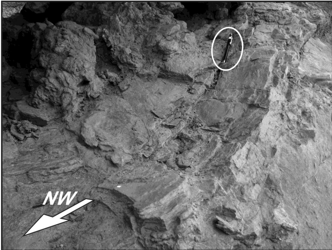
Figure 10. Ferruginized siltstone (gouge) highlights the NE -SW normal fault plane surface displacement in the sector I. Scale indicated by pen highlighted by the ellipse forming open folds in the sandstone facies Ss . The failures have directions NW- SE and ENE -WSW with dip angles of moderate to high ( 60^{\circ} - 70^{\circ} ; Sector II ) , sills facies Dm housed occur predominantly along the lodging of the AF1 and are associated with breccias facies Bi (Fig. 7C ) , as the folds exhibit inter - flaco angles between 150^{\circ} - 170^{\circ} (sector III ; Fig. 4B ) .
