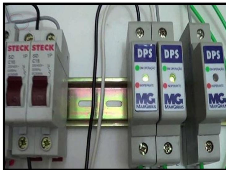
Fig.34. Painel Interno com DPS.
