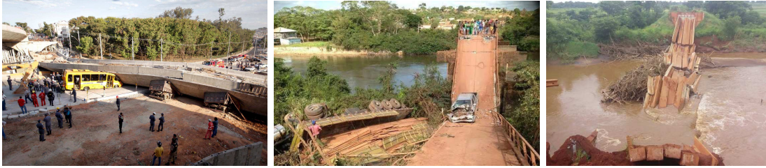
Figure 2 – Structural collapses in Brazil (from left to right): the Guararapes Battle Viaduct (Minas Gerais, 2014), the Bridge over the Aracatú River (Pará, 2014), and the Bridge over the Santo Antônio River (Mato Grosso do Sul, 2016).
