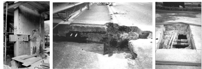
Fig. 3. Damage scenarios carried out in the Z-24 Bridge. Left to right: pier settlement, failure of anchor heads, and tendon rupture.
