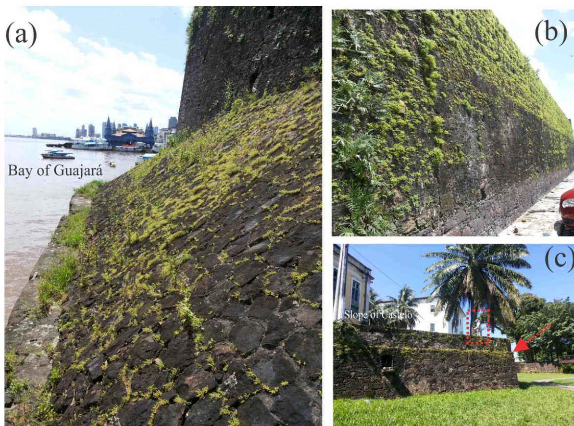
Fig. 9. Bioreceptivity in FCPB: (a) surface tilted towards the Guajar bay with vegetation at the joints between rocks; (b) wall facing the Aai Market with vegetation on the upper, this sidewalk presents accumulation of human excretory fluid (urine), which may justify less occurrence in the lower area; (c) dry moat counterscarp, with vegetation in the upper and in the horizontal shoulder, and worker in vegetation cutting procedure (red contour).
