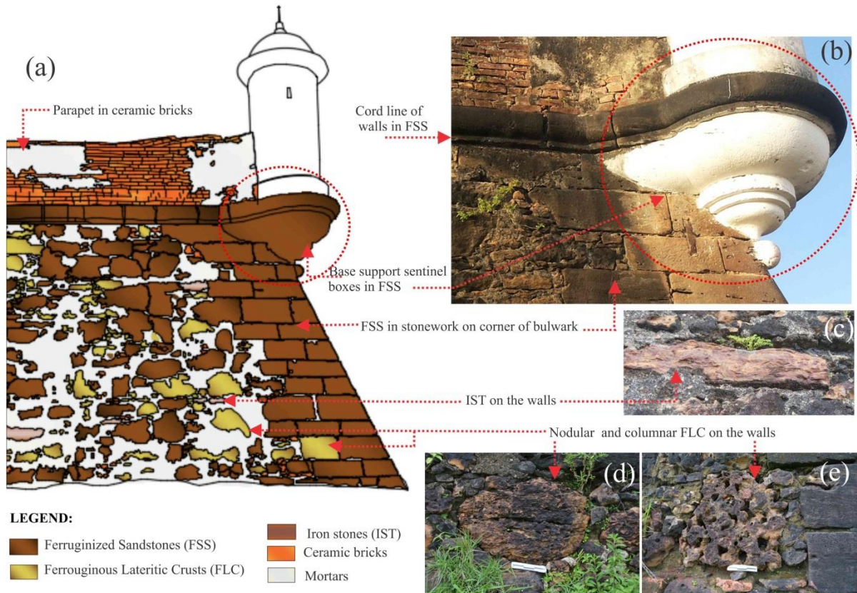
Fig. 3. (a) Face of São Pedro bulwark, exemplifying the FSS predominance from the base, corners bastions until the cord line of walls and to a lesser extent scale FLC's and IST's blocks, ceramic bricks and remnants of laying mortars; (b) Detail of base sentinel boxes (whitewashed), cord line and faceted corners in FSS; (c) IST on the walls; (d) Nodular/cavernous FLC on the walls; (e) columnar/tubular FLC (lying down) on faces of N.Sr a da Conceição bulwark.
