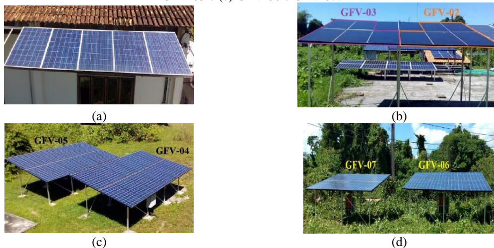
Figura 1.20 – Sistemas FV implantados no âmbito do LSHM: (a) GFV-01, (b) GFV-02 e GFV-03, (c) GFV-04 e GFV-05 e (e) GFV-06 e GFV-07.
