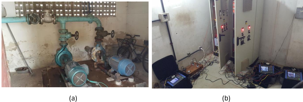
Figure 7-9 – Pumping System at the Federal University of Pará: (a) 15 kW SCIM and (b) Power quality analyzer for electric motors consumption measurement.
